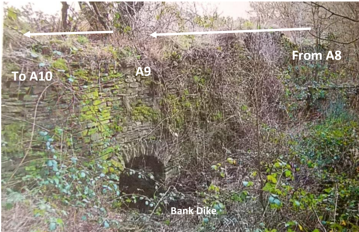
29. Culvert carrying Bank Dike beneath Meltham 70 at point A9. This 'bridge' is referred to in various User Evidence Forms. Photo supplied by Applicant 1 in Jan 2016.
