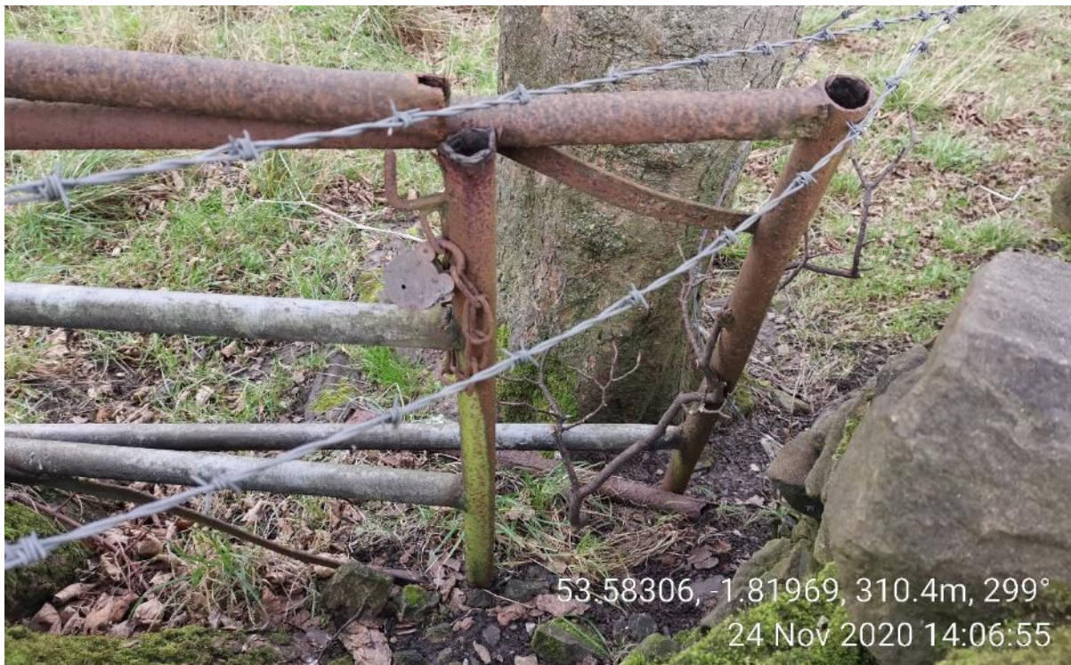
6. Close up of dilapidated gates in field near point A, showing lock and chain. 24 Nov 2020.
